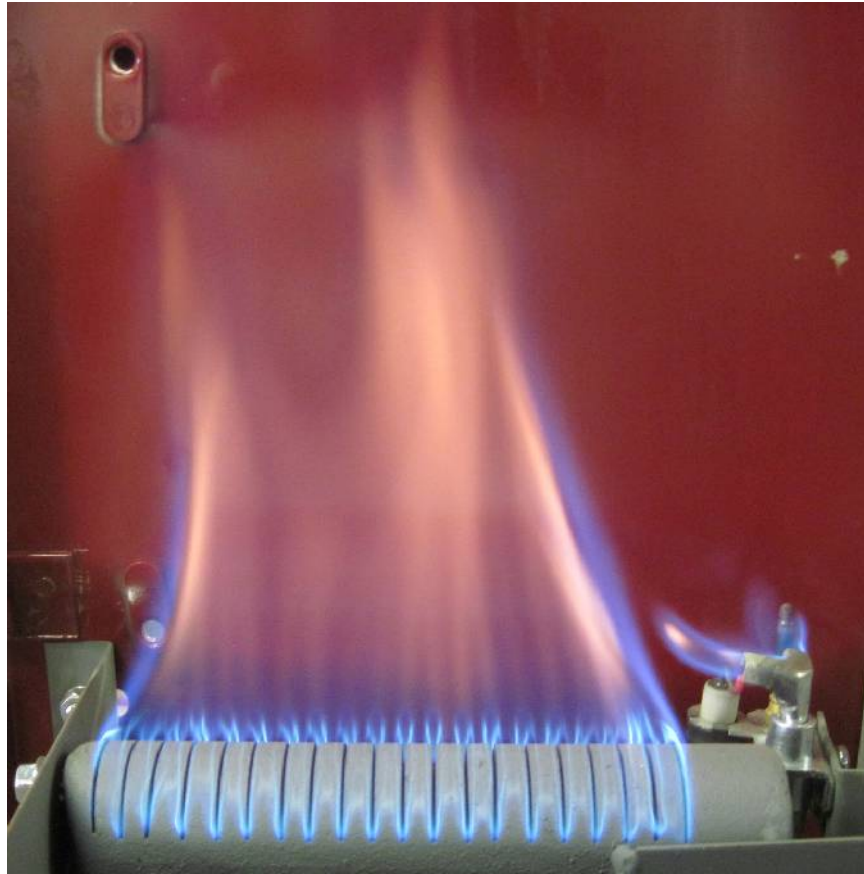
Illustration 4: Burner with Insufficient Air
